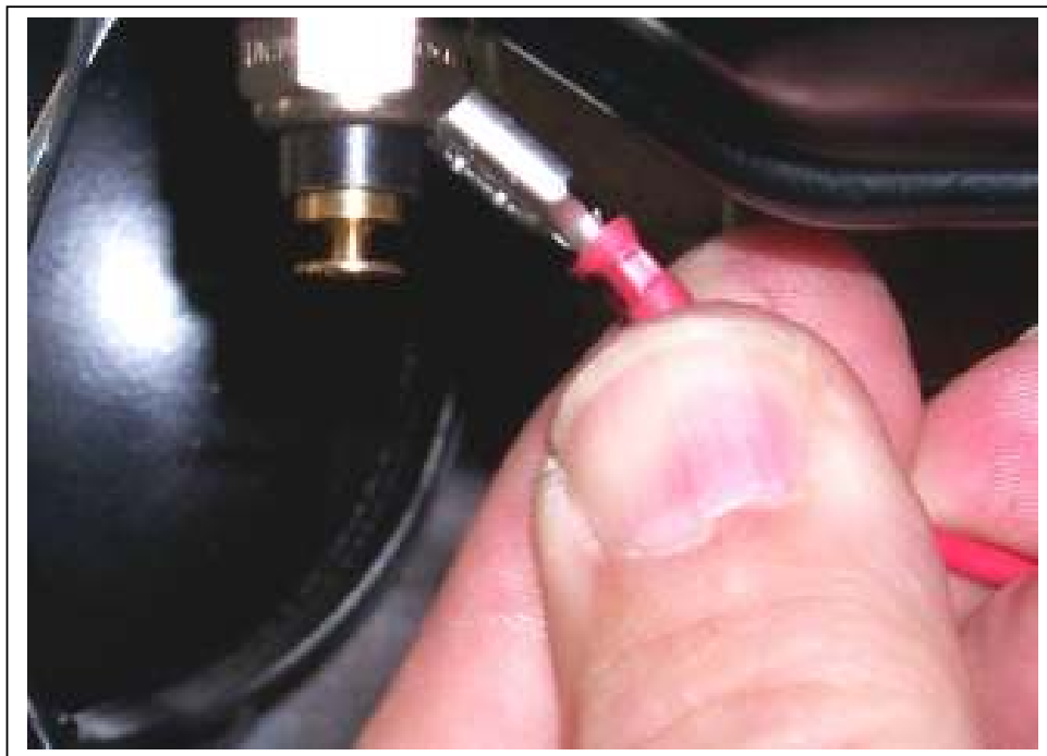
Figure 65 Earthing of CHT Sender, to check the wire to the SkyDAT.
